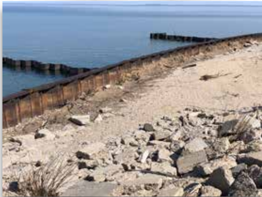
Evidence of SPS damage on the north side of the Lighthouse.
