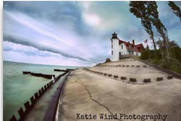
The Lighthouse "apron" showing signs of wear and tear.
